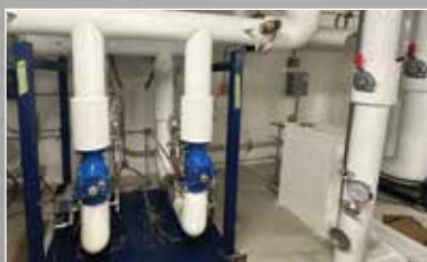
Mechanical Insulation and National Model Codes
